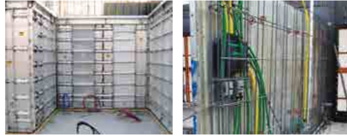
+2 Installation of electrical, plumbing components and steel rebar. Installation of I/C and wall panels
